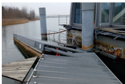
Fig. 1. A damaged accessway to a floating house in the marina of Geerswalde
