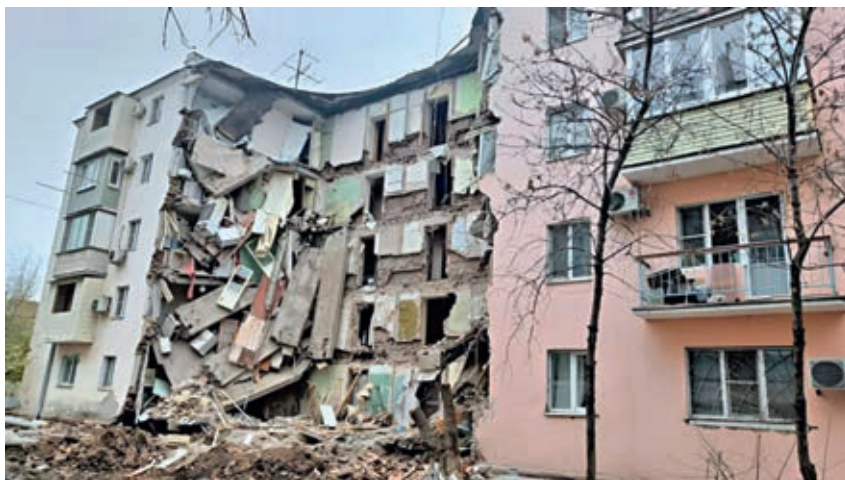
Fig. 5. General view of a destroyed apartment building in the Leninsky district on 1a Vokzalnaya Square in the city of Astrakhan
