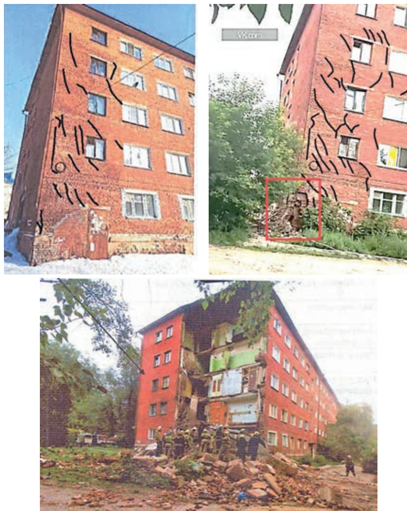
Fig. 4. General view of an apartment building in XX Partsezda St. in Omsk before and after the collapse (the arrow shows the progressive destruction of the corner section of the outer wall a few seconds before the collapse of the end part of the building)
