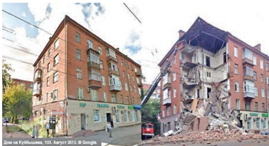
Fig. 1. General view of an apartment building in Kuibyshev Street in Perm before and after the collapse
