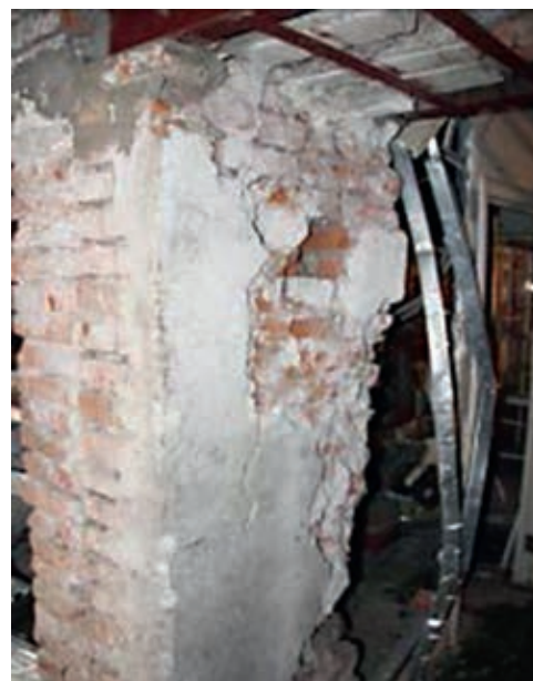
Fig. 2. View of the pillar of the non-designed opening in the basement, which was the source for activating the process of destruction of the building (the state of the pillar, recorded before the collapse of the corner of the building)
