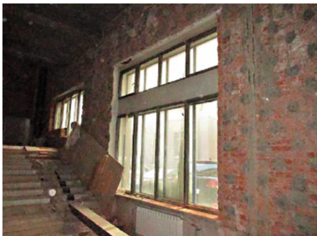
Fig. 7. The masonry mortar weathering, local damage to the brickwork of the walls on the first floor
