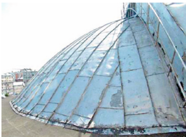
Fig. 8. Deformation, mechanical damages, corrosion, reduced tightness of metal sheet seam fasteners on the building's dome roofing
